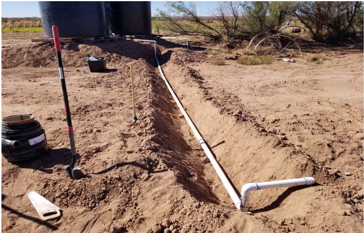
Figure 2: The subsurface PVC line connecting the tanks to the drip irrigation. Leupp, AZ. 2019
